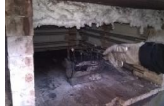
Gambar 3. Tungku proses hot dip galvanizing
